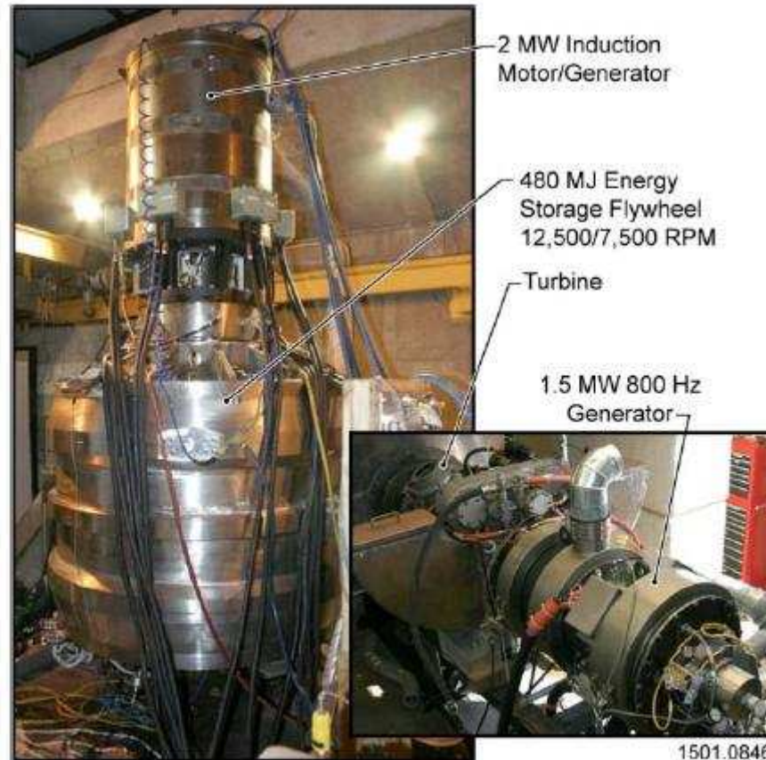
Partial Views of the Inside of the Bunker Showing the Flywheel Energy Storage System and the High Speed Generator
