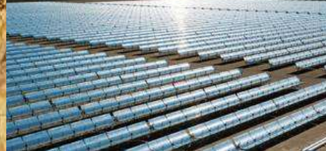
Nevada Solar One 64 MW Boulder City, Nevada
